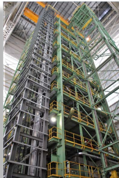
Bright Anneal line construction
